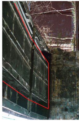
Metal casing containing six 400kV cables (within the red line), Kingsland Basin footbridge. (See also above right)
