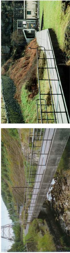
Surface troughing crossing the river Etherow and entering the Woodhead tunnels (carrying six 400kV cables - a doubling circuit)
